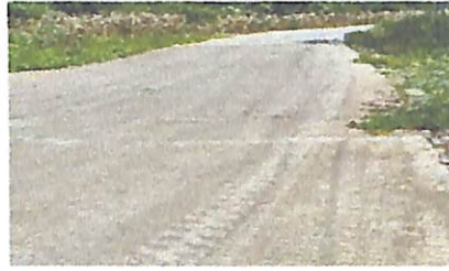
Figure 4. Road condition to Pencong Hot Springs
